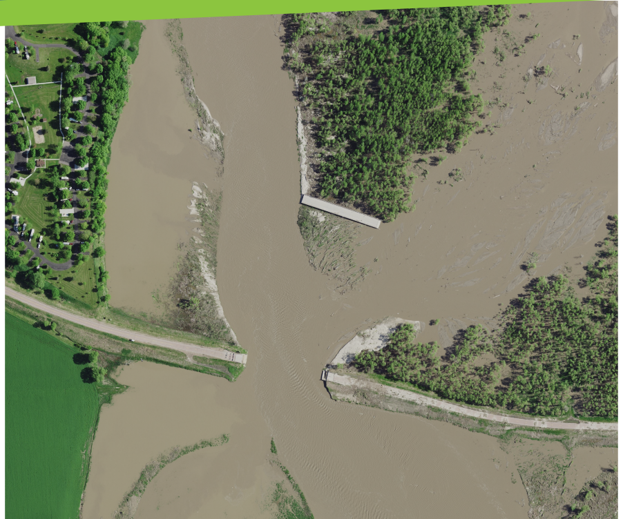
Displaced bridge in USGS/FEMA flooding imagery
